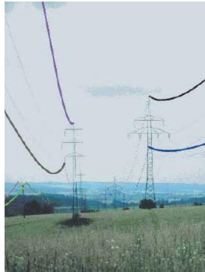
Figure 9 Fiber-in-Gas installation (Source: SEMPRA Fiber Links) and fiber over power lines (Source: ALCATEL solutions)
